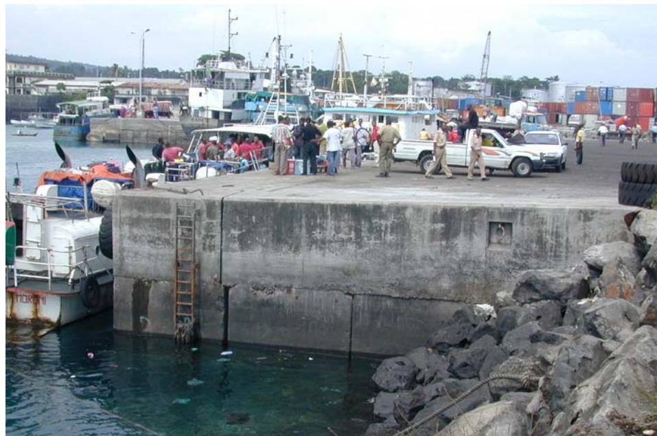
Figure 12 : View of the new pier of the port of Moroni (at left behind, the old first pier of the port) There is not enough water depth to install the tide gauge here and the concrete blocks are collapsing into water
