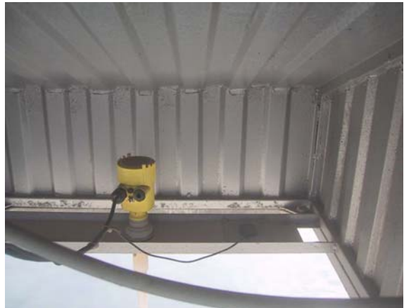
Figure 21, VegaPuls Radar Sensor (yellow) and GPS Patch Antenna alongside at the open base of the galvanised steel cabinet. The microwave / radar antenna wave-guide extends (approx 35cm) below the VegaPuls sensor.
